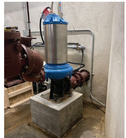
After installation of envie 3 pump
